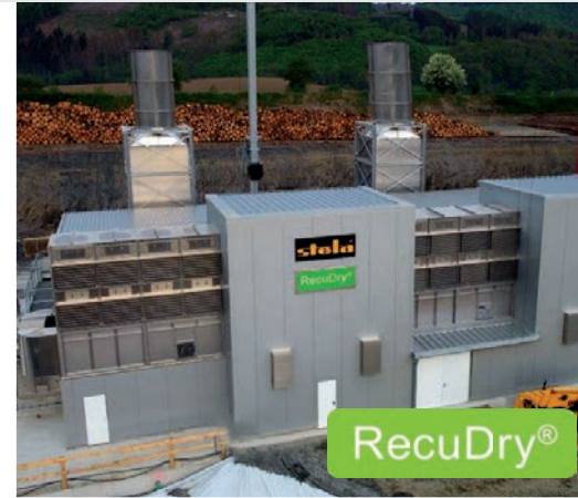
Pieper Pellet GmbH, Germany
